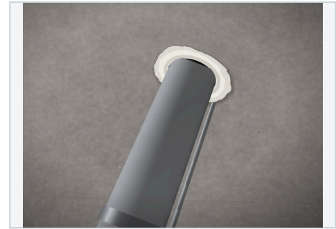
Photo 3 — Third-floor riser: soil pipe with no collar
