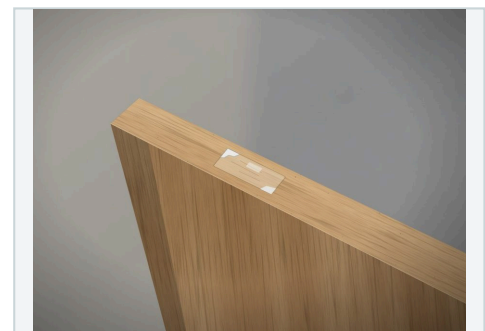
Photo 5 — Riser cupboard door: no legible labelling
