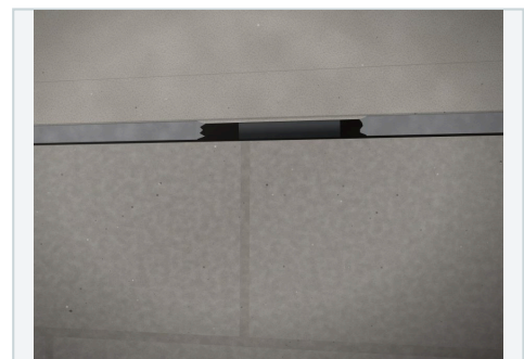
Photo 1 — Electrical intake room: joint seal missing at the head
